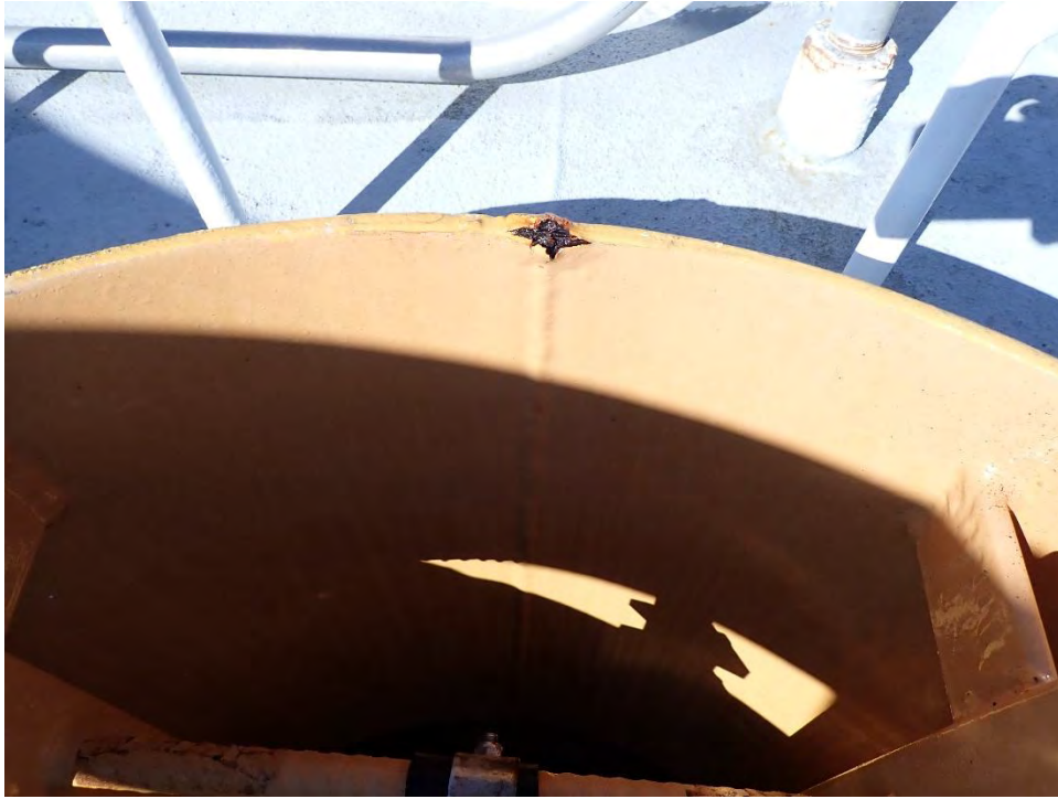
Photo 9: Roof hatch with corrosion
