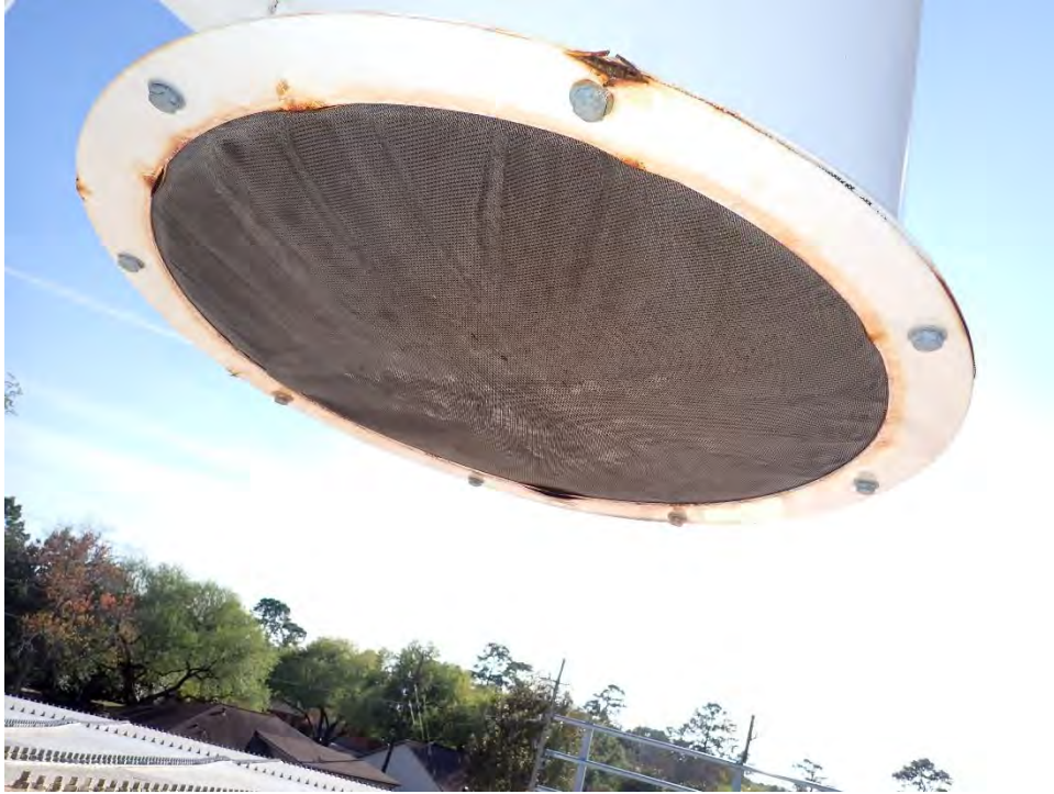
Photo 9: Roof vent with corrosion
