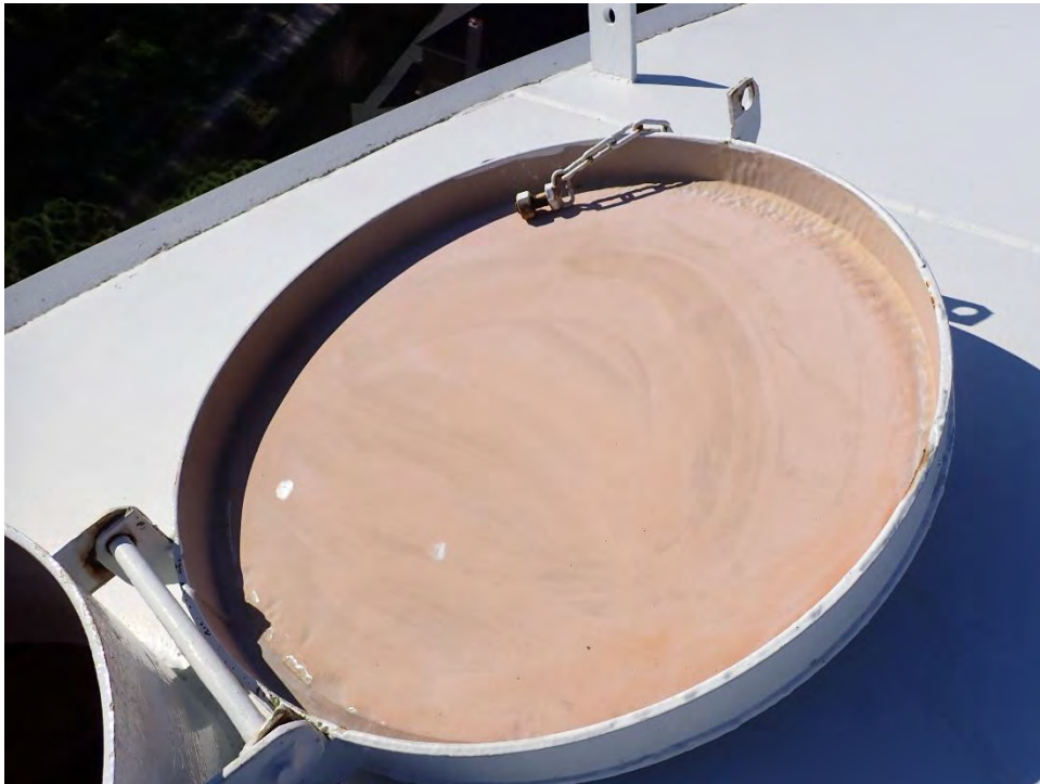
Photo 6: Roof hatch with missing gasket material and corrosion
