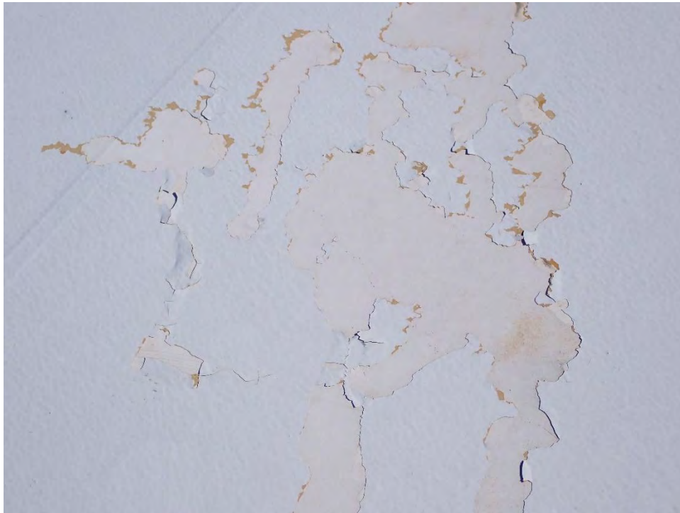
Photo 5: Roof with coating delamination
