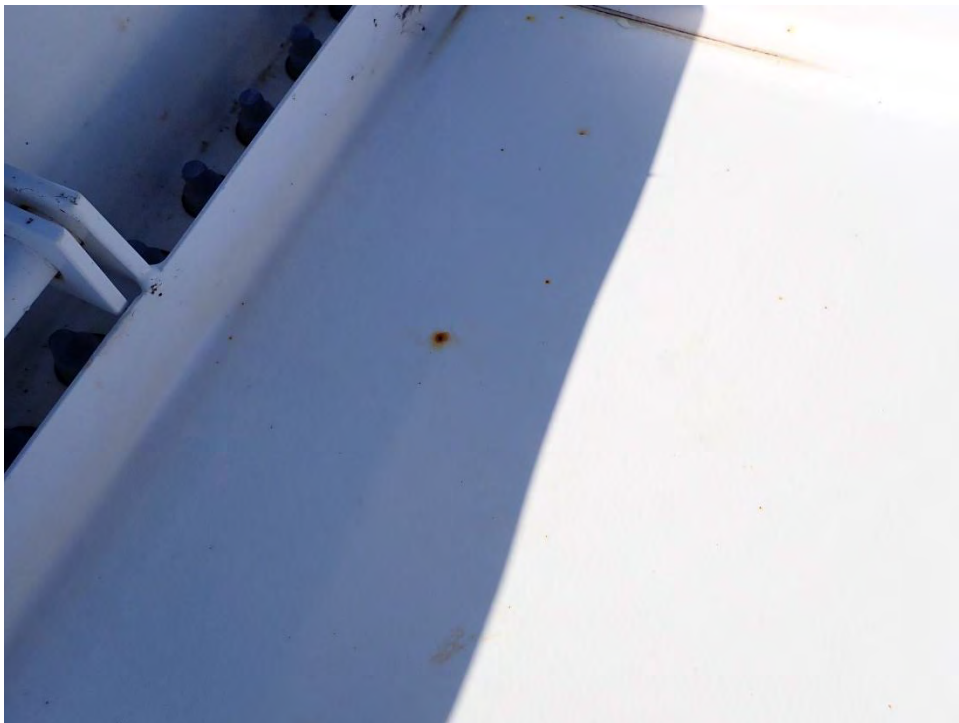
Photo 10: Roof hatch with corrosion
