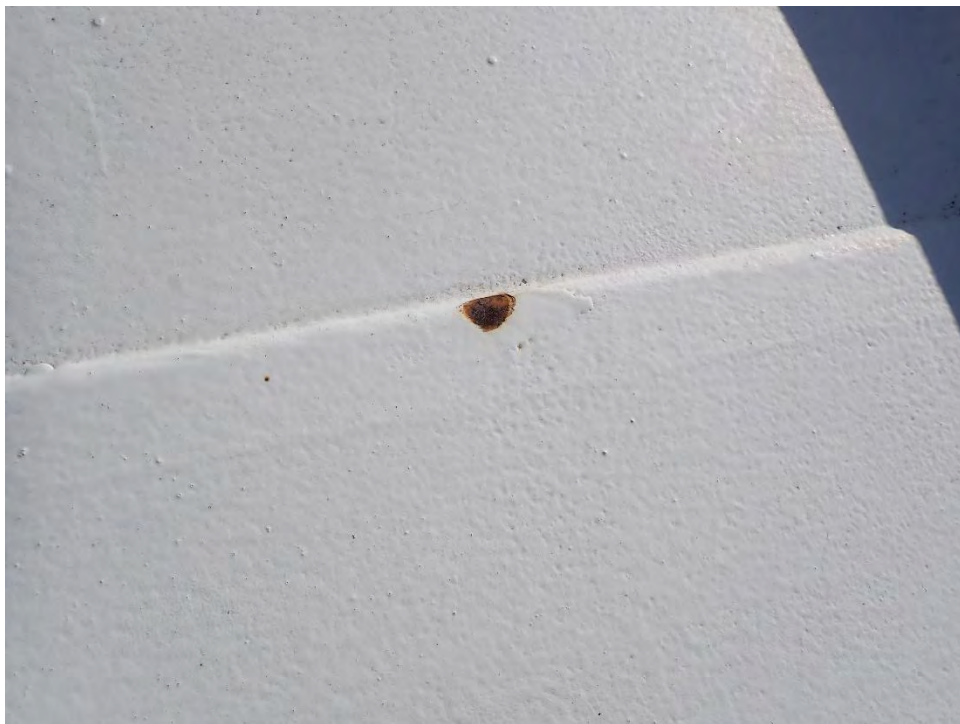
Photo 4: Roof with corrosion
