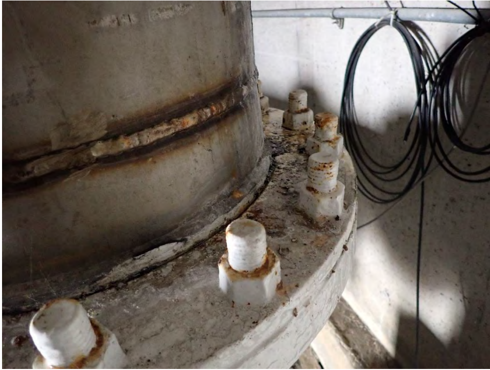
Photo 9: Pedestal piping with corrosion
