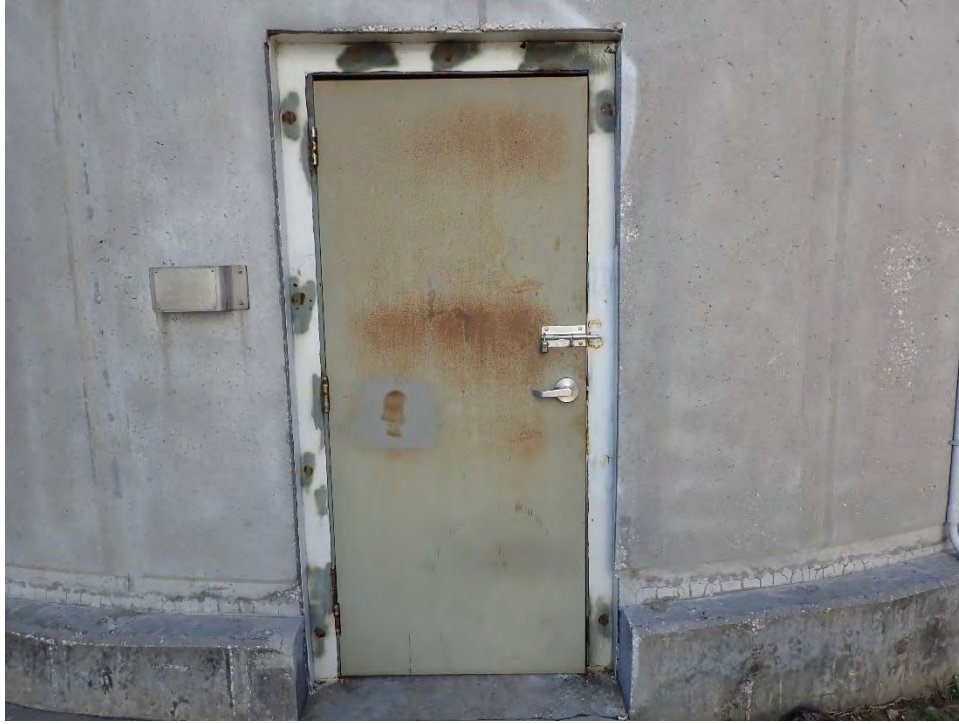
Photo 1: Door with corrosion
