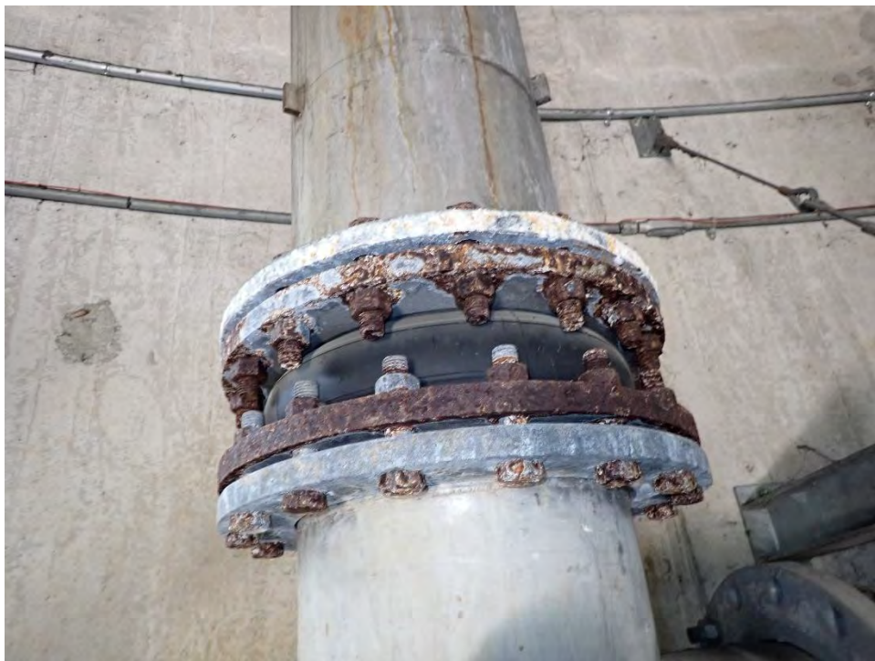
Photo 12: Interior pedestal piping with corrosion
