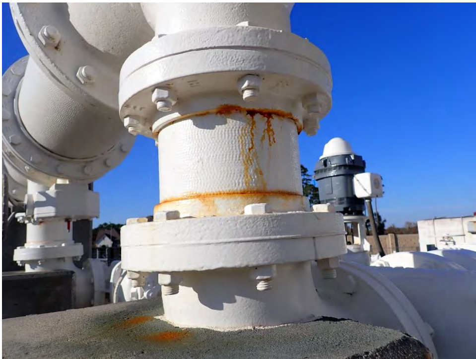
Photo 6: Yard piping with corrosion
