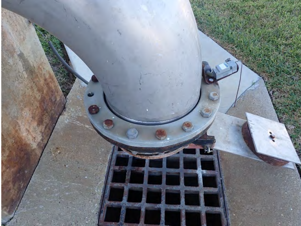
Photo 1: Drain piping with corrosion
