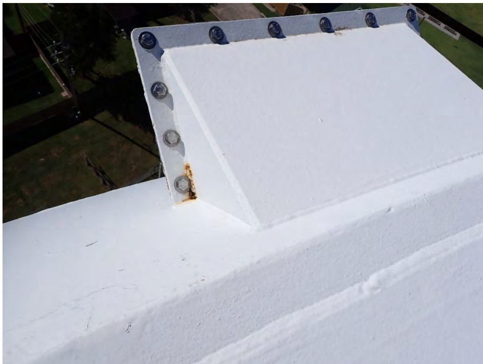
Photo 8: Shell vent with corrosion
