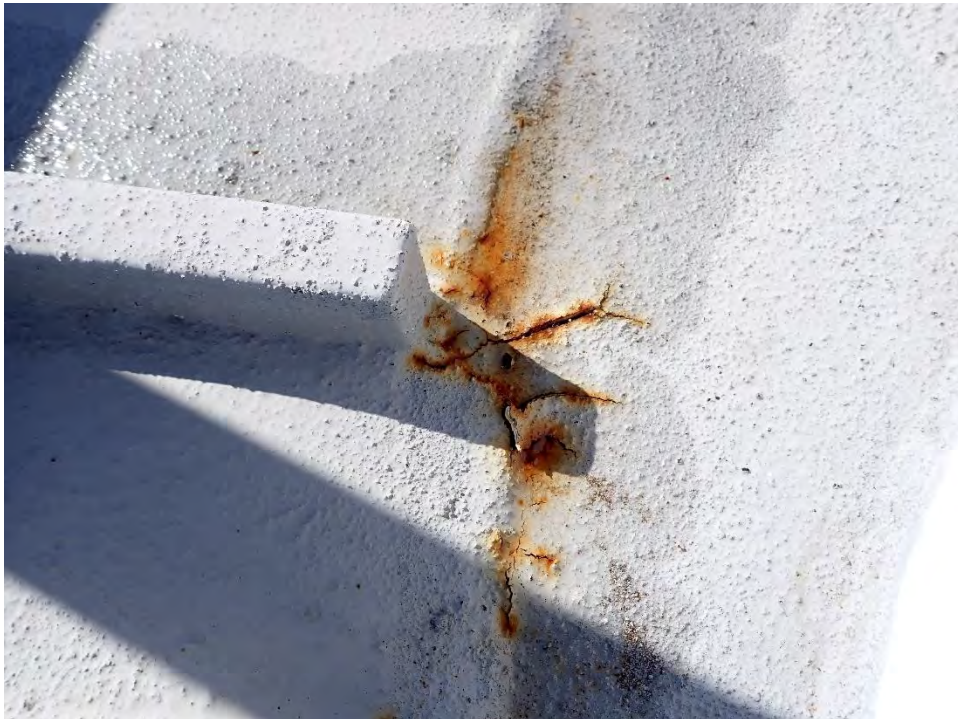
Photo 2: Roof with corrosion
