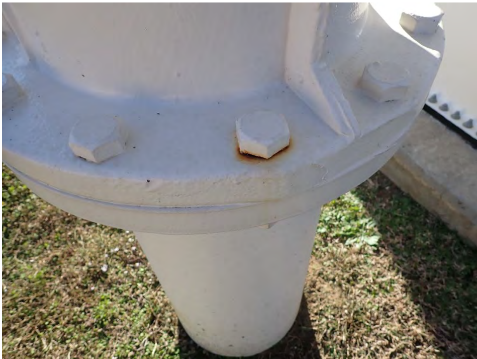
Photo 4: Tank piping with corrosion
