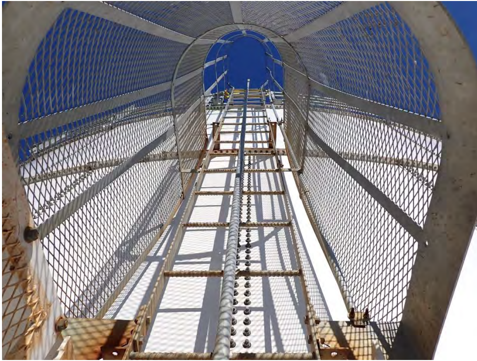
Photo 7: Safety cage with corrosion
