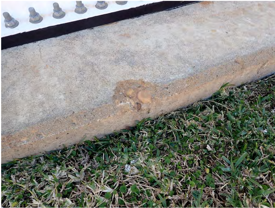
Photo 1: Foundation with spalling
