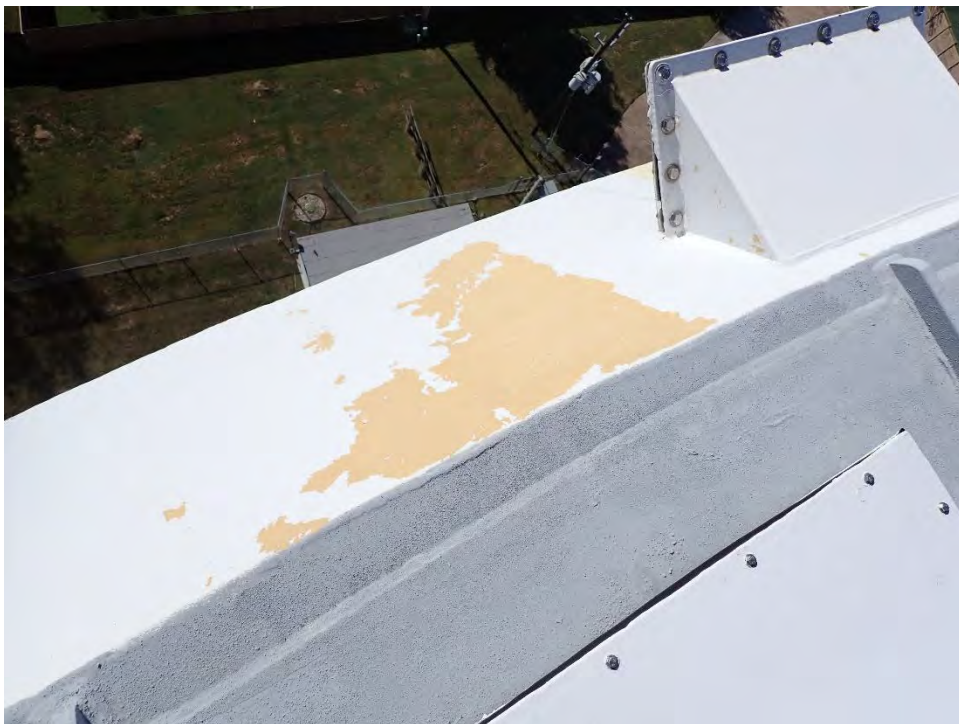
Photo 4: Roof with coating delamination
