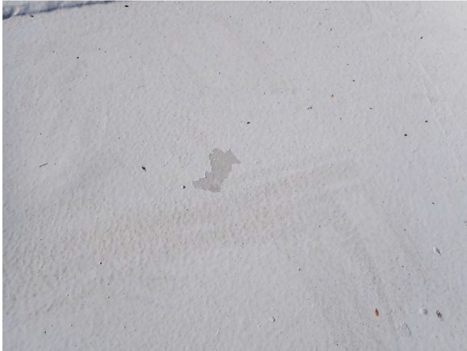
Photo 3: Roof with topcoat delamination
