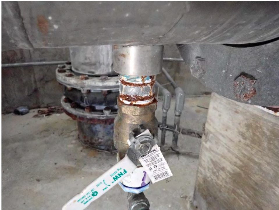
Photo 11: Interior pedestal piping with corrosion
