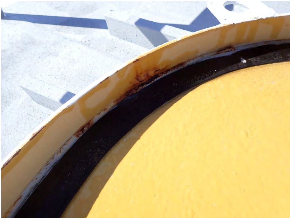
Photo 10: Roof hatch with corrosion
