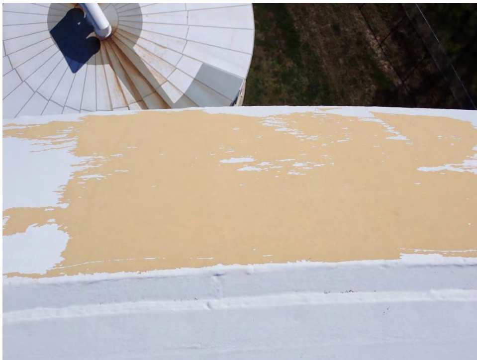
Photo 6: Roof with coating delamination
