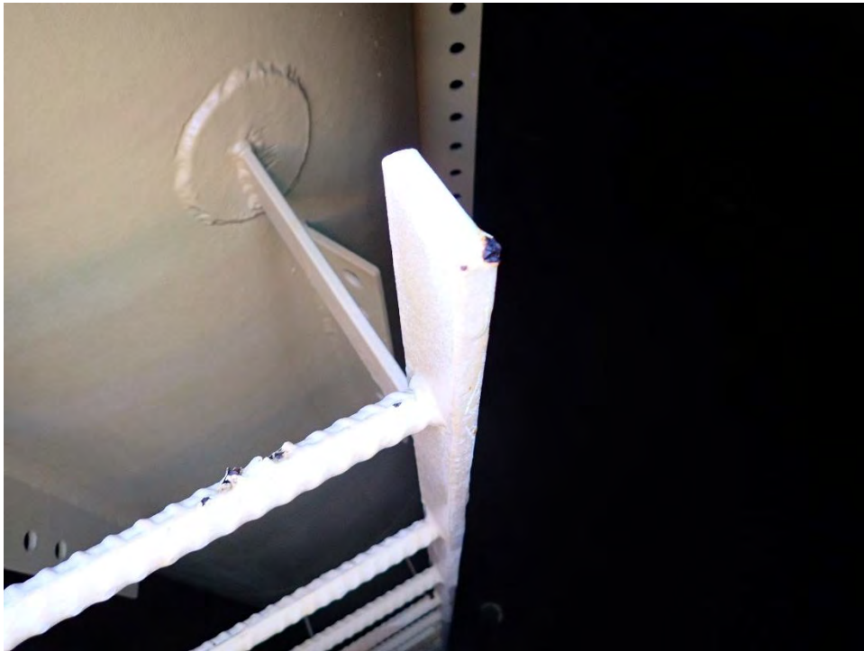
Photo 10: Wet bowl ladder with corrosion
