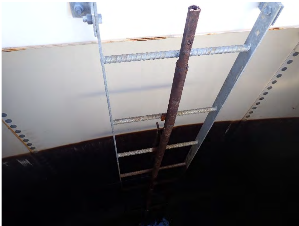
Photo 12: Ladder with corrosion
