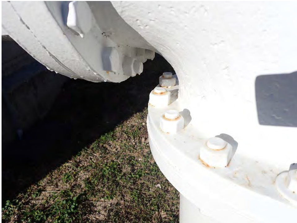
Photo 2: Piping with corrosion
