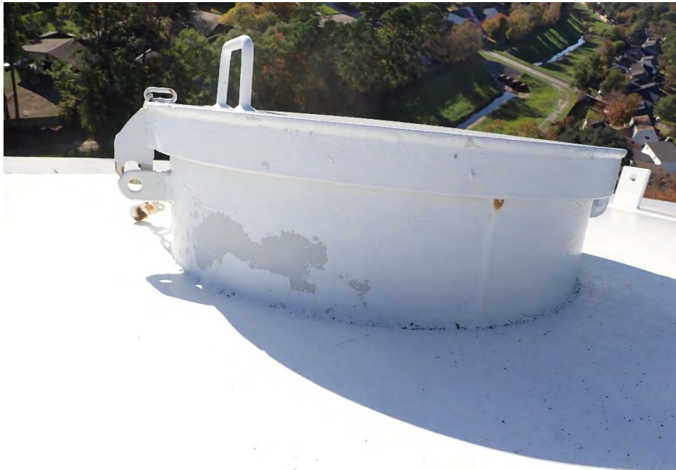
Photo 8: Roof hatch with corrosion
