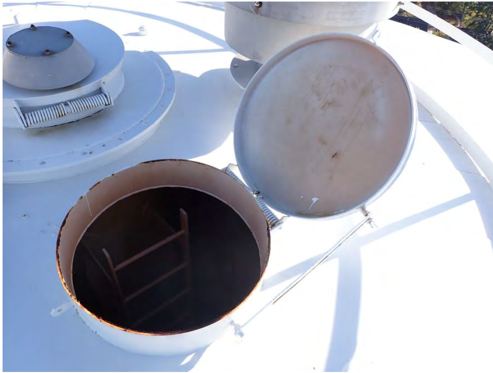
Photo 7: Roof hatch with corrosion and missing gasket material
