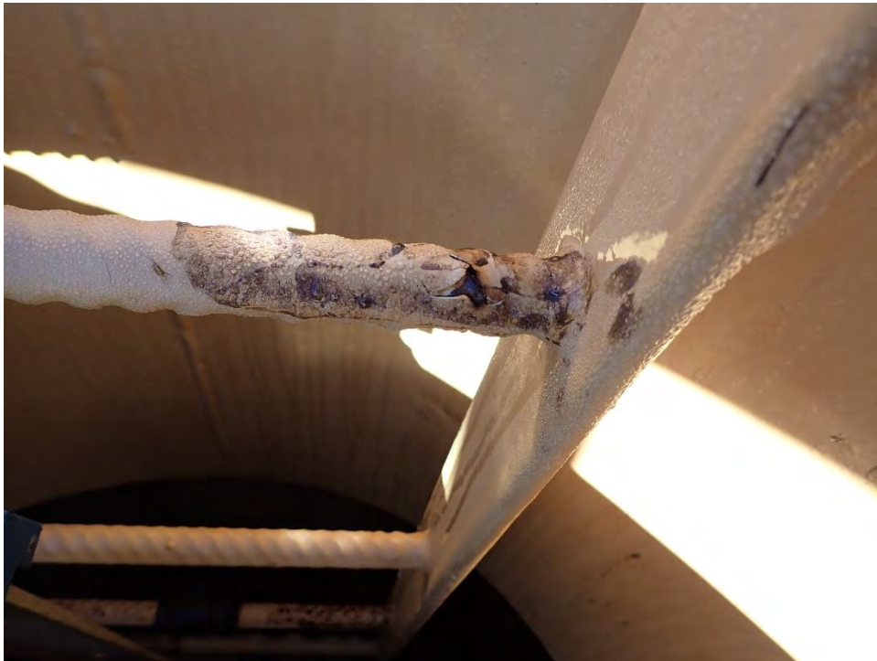
Photo 14: Wet bowl ladder with corrosion
