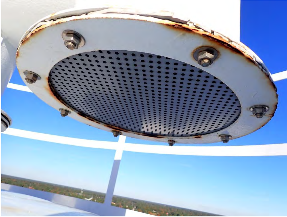
Photo 5: Roof vent with corrosion
