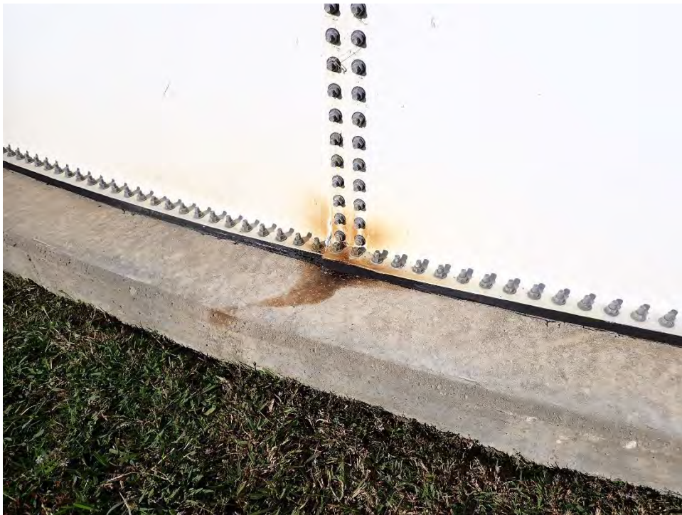
Photo 2: Tank wall with corrosion
