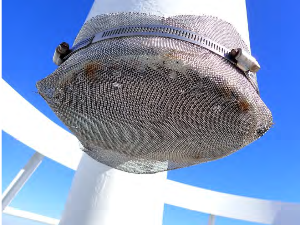
Photo 7: Roof vent with corrosion
