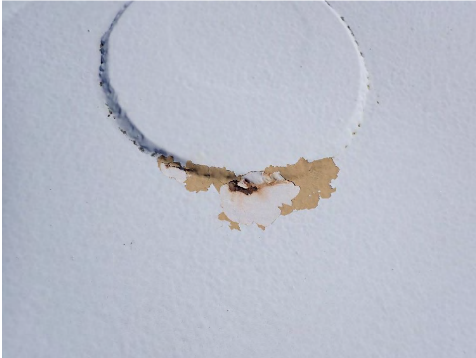
Photo 3: Roof with topcoat delamination and corrosion
